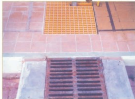
Corroded Steel Grating Vs GRP Moulded Grating
